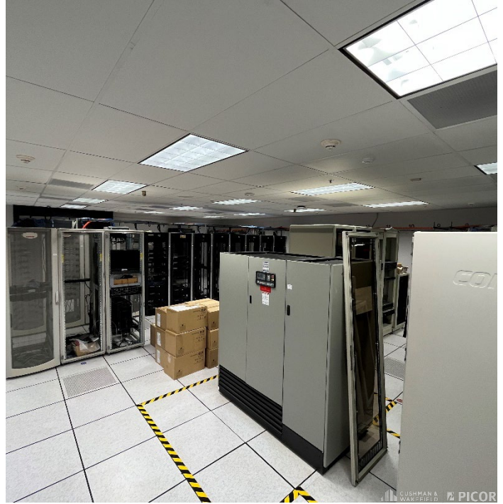
IT Room – Raised Floor
