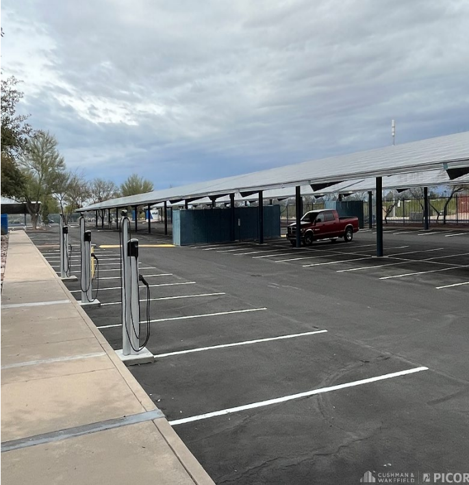
EV Charging Stations and Solar Panels
