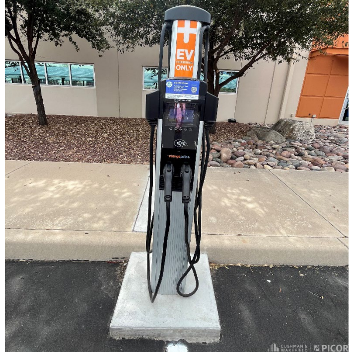
Three Level 2 EV Charging Station
