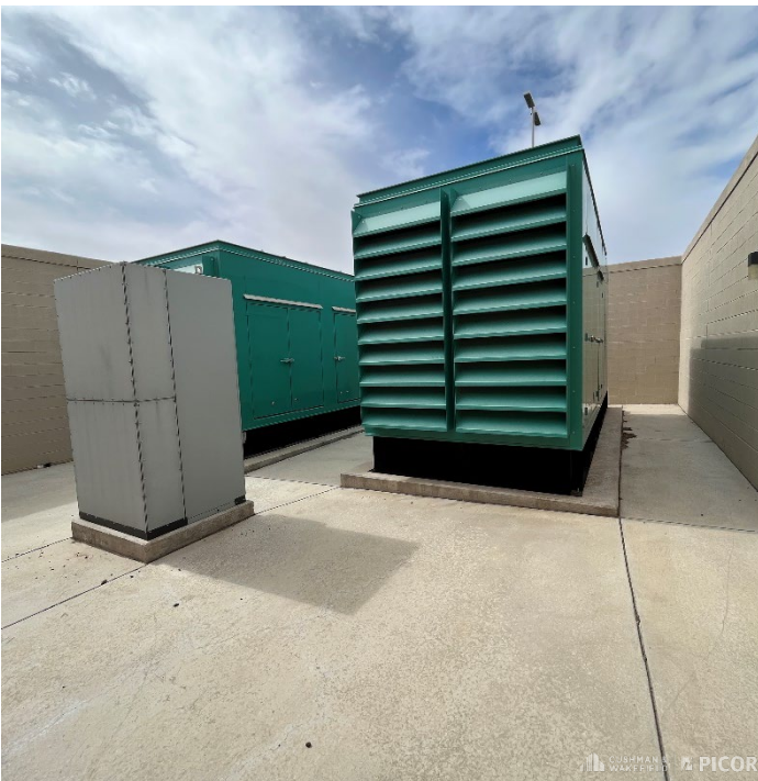
Generators – Redundant Auto-Transfer System
